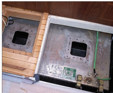
Fuel tank inspection ports are essential for monitoring diesel quality and condition. There must be one port in each baffled chamber of a connected fuel tank to allow thorough cleaning after contamination with bad fuel or bacteria.
