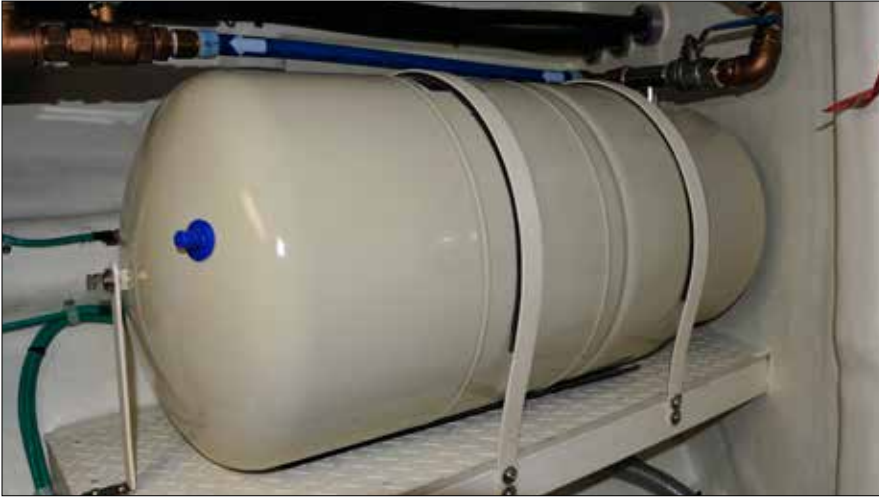
Large tanks full of water are heavy and can become dangerous missiles in rough seas. This accumulator tank is properly mounted and secured with straps that encircle the unit.
