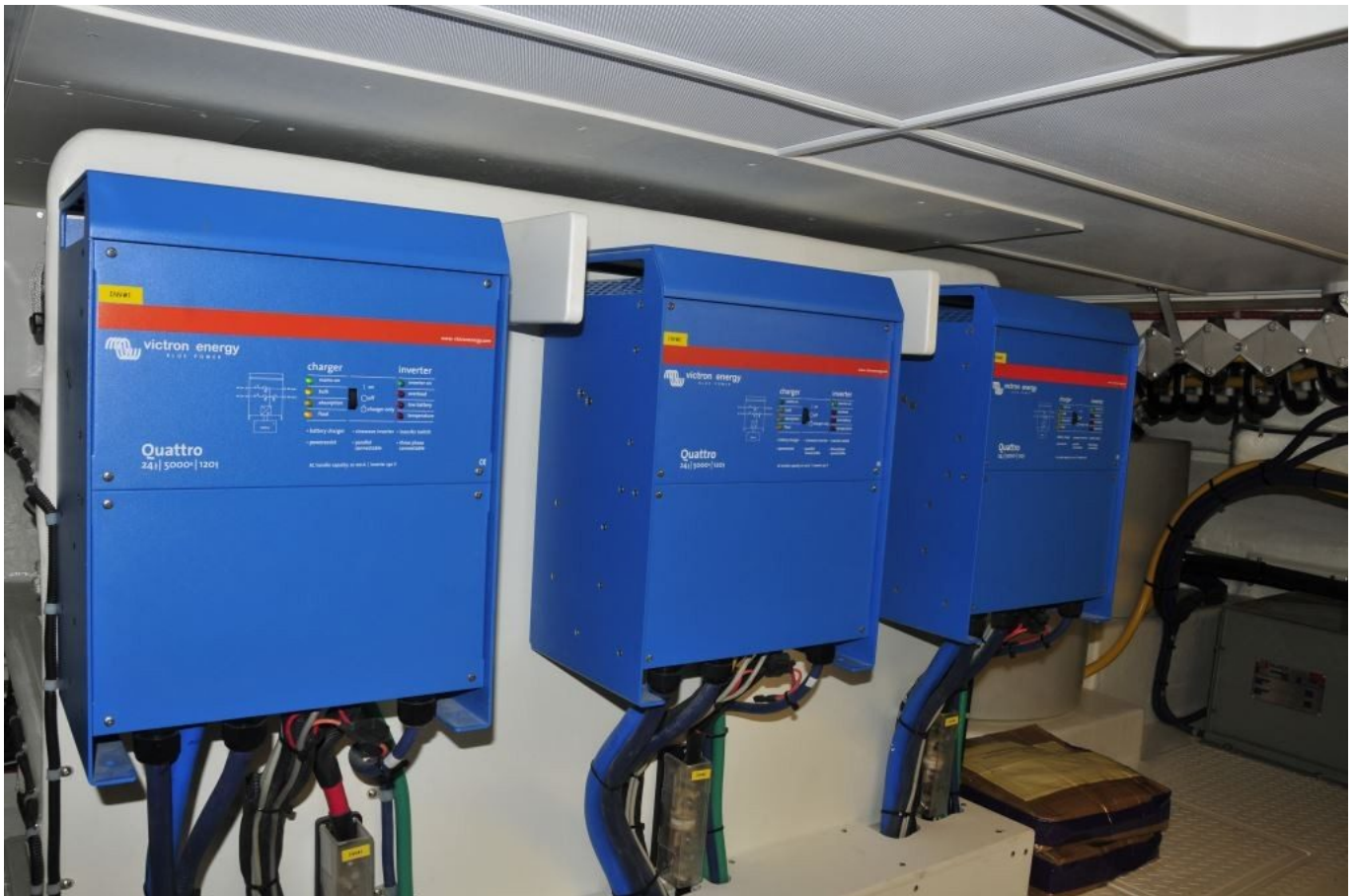
This large inverter bank supplies power to this vessel's AC
