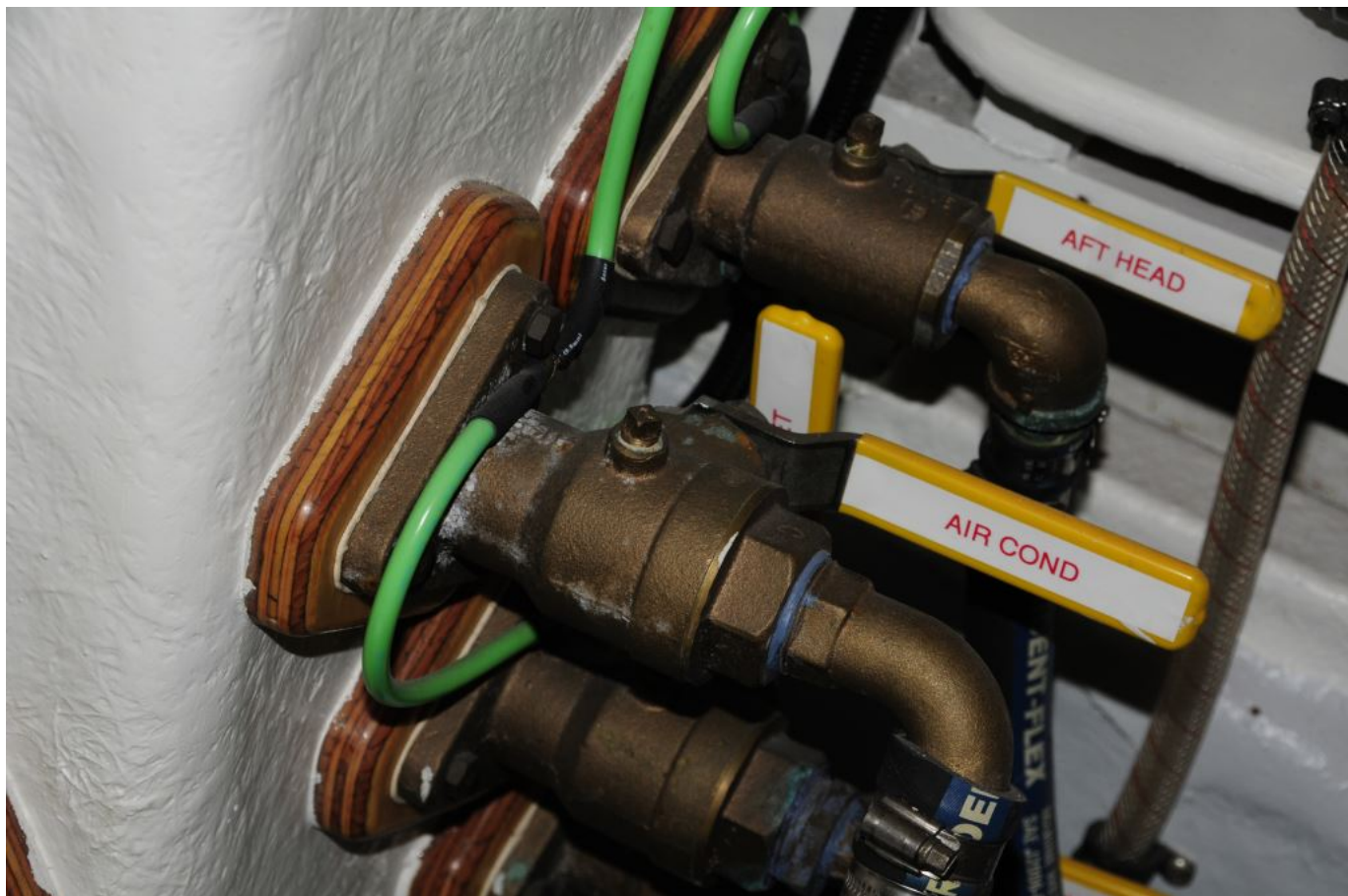
Seacocks should be accessible, without the need for tools,
