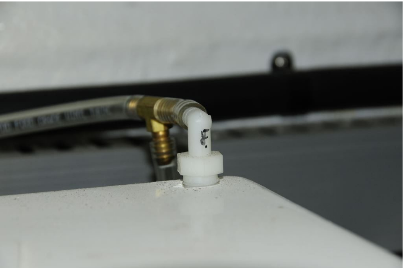
This battery box has been equipped with a remote ventilation
