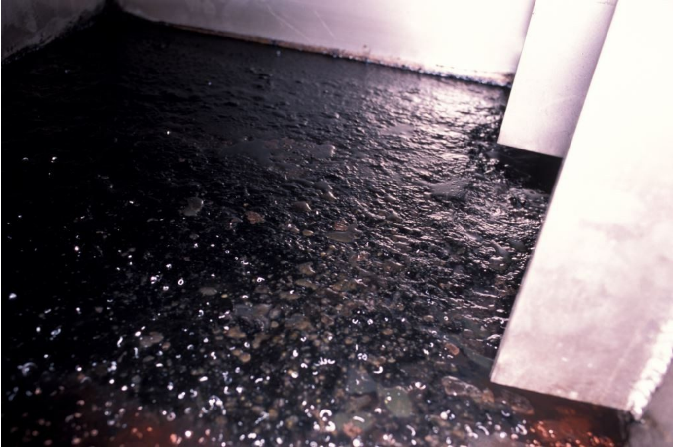
A heavily contaminated fuel tank bottom, viewed from an inspection port.
