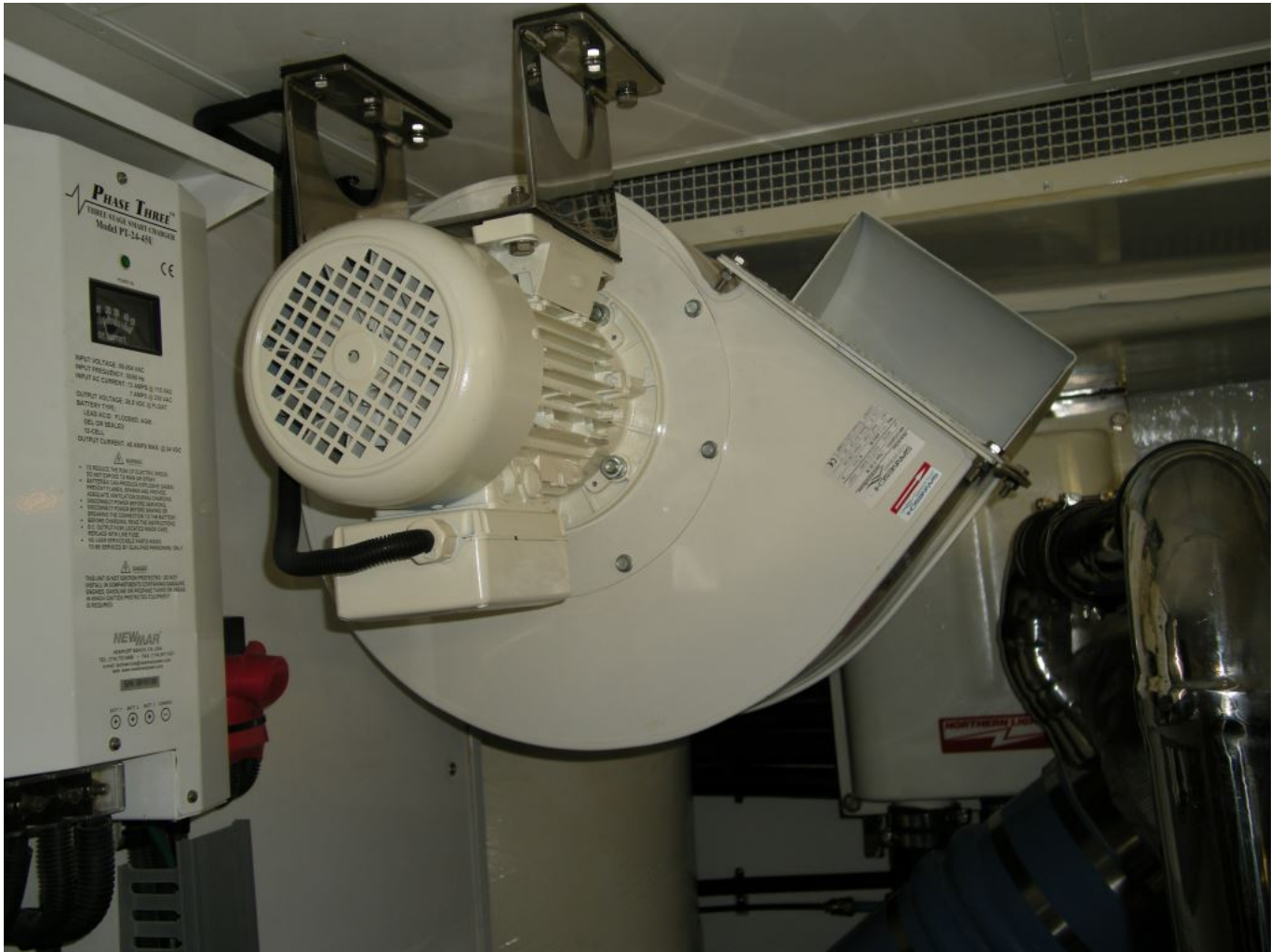
An industrial-size 'squirrel cage' blower. Units like these are designed to operate continuously, while at rest or underway.
