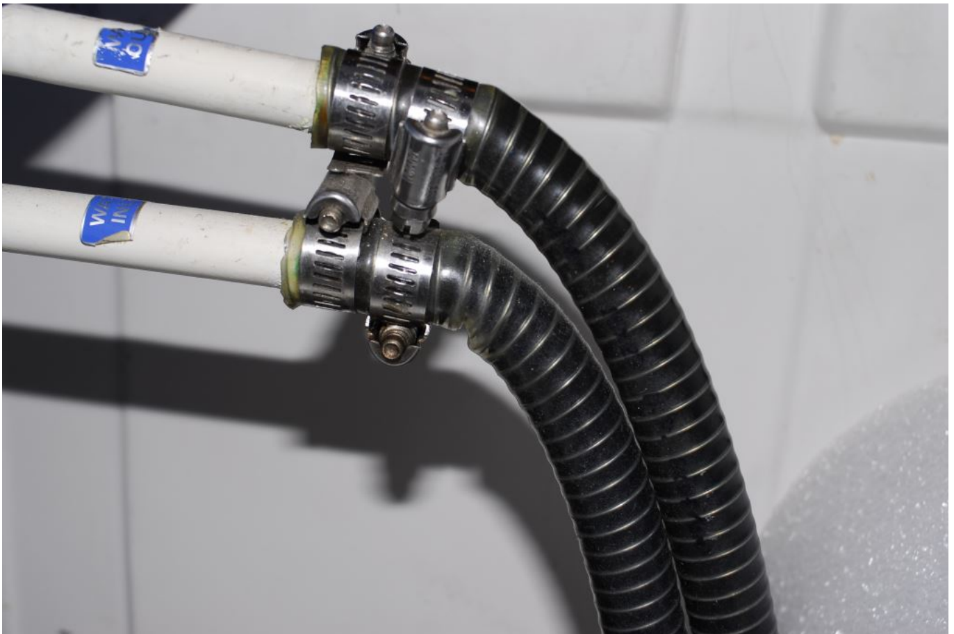
This PVC "spring hose" is unsupported, and on the verge of failure.
