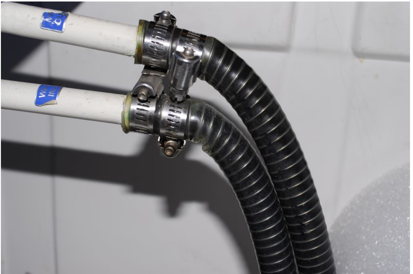
This PVC "spring hose" is unsupported, and on the verge of failure.
