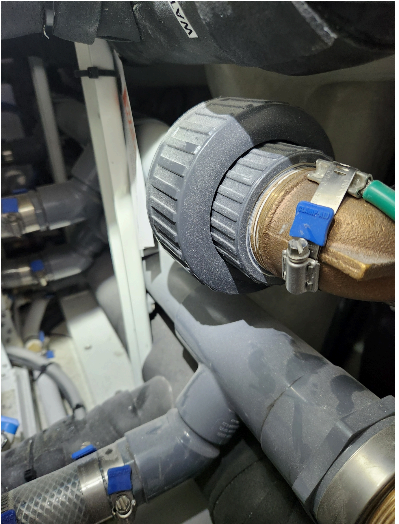
Schedule 80, heavy-wall PVC pipe, is often used by marine HVAC manufacturers for raw water manifolds, note the bracket
