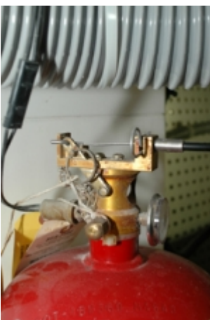
A manual T handle discharge along with the pilot light panel and override switch.
