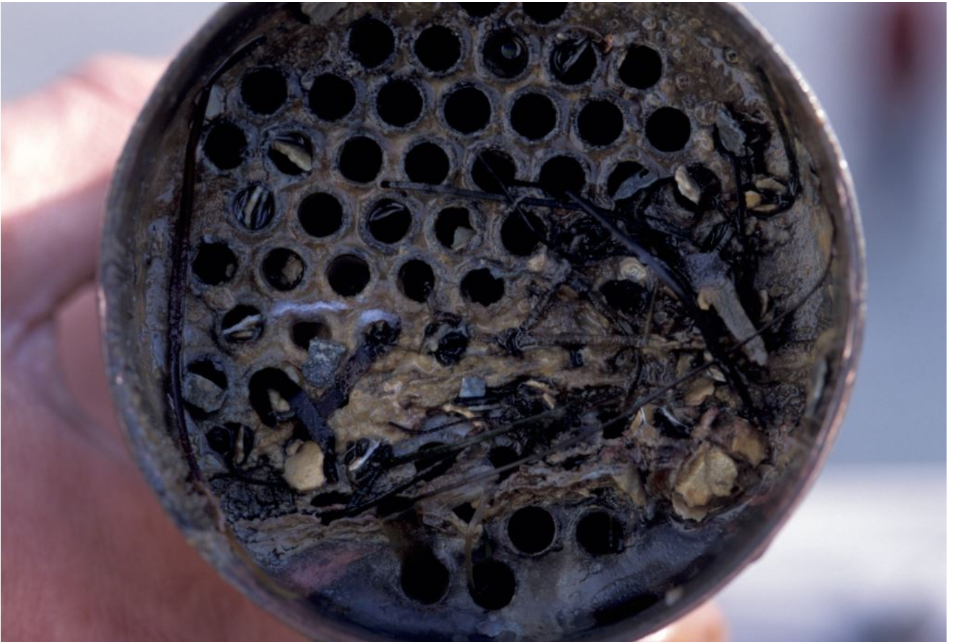
Heat exchangers should be inspected for debris accumulation
