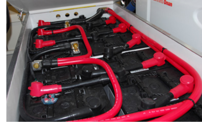
Large house battery banks require careful attention where wiring and over-current protection are concerned. Note the gaps between these batteries for heat dissipation purposes.
