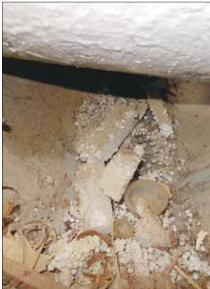
Bilge pumps are not designed to deal with the trash, dirt, or hair that can accumulate in bilges. A pump may also be fouled by new-boat detritus: fiberglass shards, wood chips, wire-ties, screws, foam, and wire insulation trimmings. The need for clean bilges is about more than just good housekeeping.
