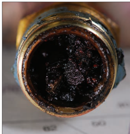
Some end-users of biodiesel report the need to change filters more frequently, at least initially. In heavily contaminated tanks, debris may lodge in fuel lines and fittings (such as the one shown here), valves, and other plumbing.
