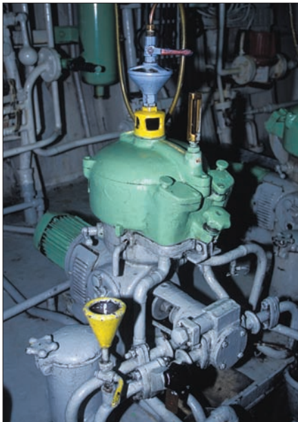
A 40-year-old centrifugal separator. It's still going strong aboard an expedition cruise ship that operates from Arctic to Antarctic waters, where fuel filtration is critical but the nearest spare filter-element may be thousands of miles away.
