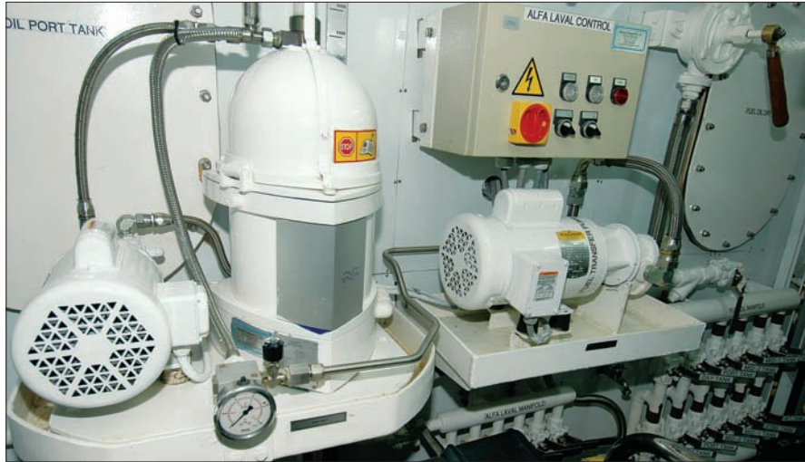
An Alfa Laval separator—installed aboard a 65'/19.8m motoryacht—is plumbed via a manifold to each of the vessel's tanks, and polishes fuel before any is pumped to a day tank.
