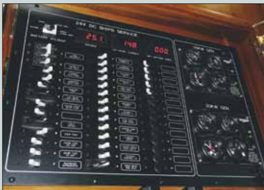
This easy-to-read panel for the ship's 24VDC system belies the unavoidable complexity in an electrical system for a vessel of this size and capability.
