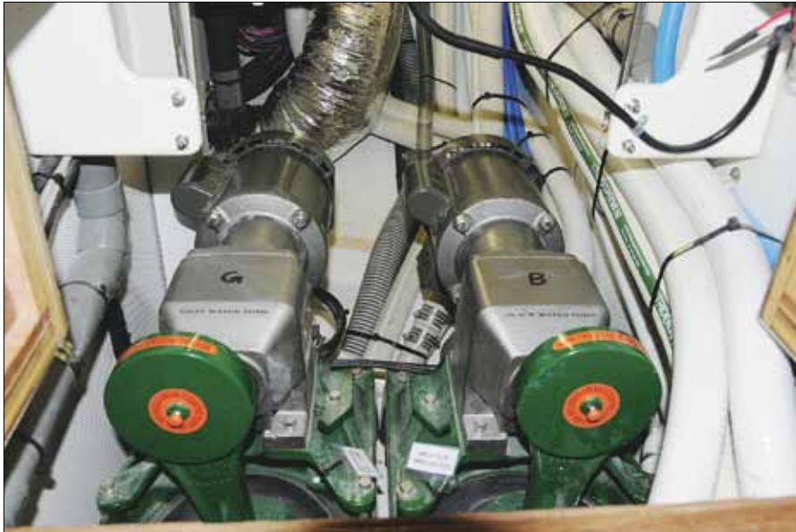
For smart redundancy, these two pumps serving black- and gray-water tanks, are identical; and by simply manipulating a set of valves, either one can be used for either application.
