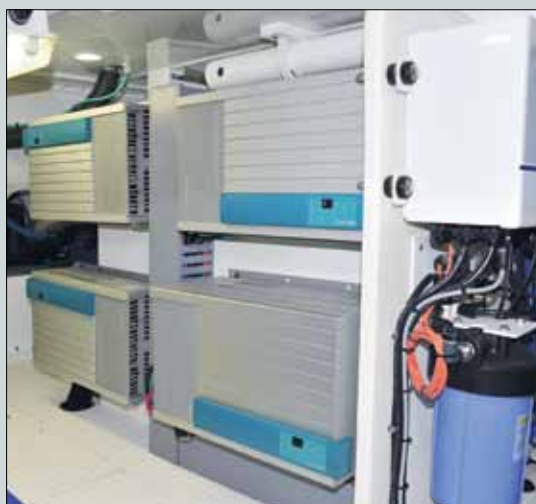
The large house battery bank is charged through four integrated 100 amps, 24V temperature-compensated battery chargers delivering ample charge capacity.
