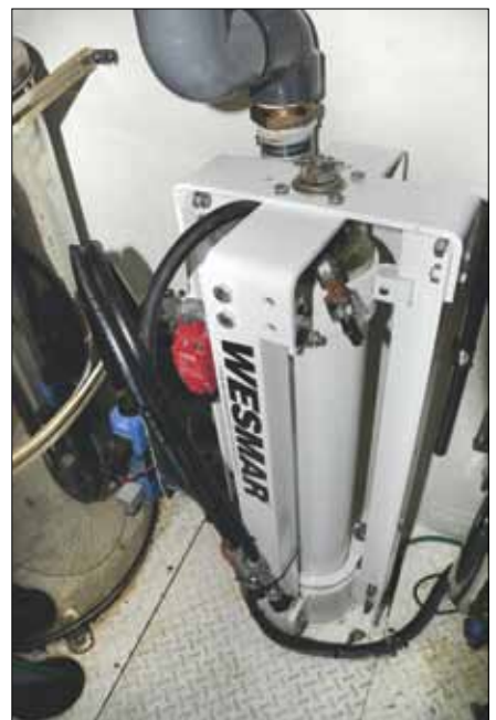
The sonar transducer is easily accessible for regular inspection and maintenance.
