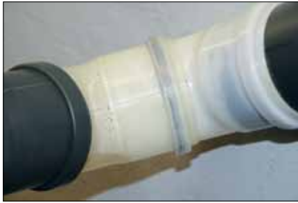
Little heat goes to waste. Here, a test unit exhaust is piped through simple plastic tubing through which condensing water is visible.
