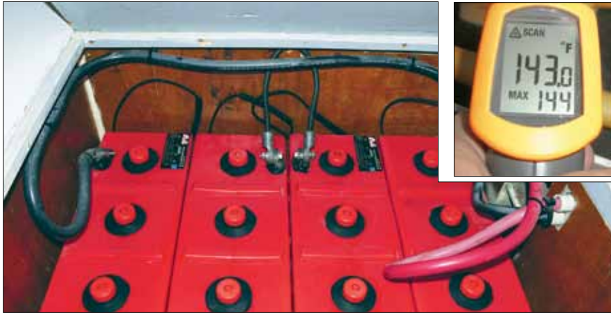
Batteries tightly stacked "sandwich" style can overheat because no air can circulate around those in the middle. The center batteries in this bank are noticeably hotter than those on the perimeter. Also, the locker is resin-coated wood, and the top of the space is not ventilated. This compartment would benefit from a re-design.
