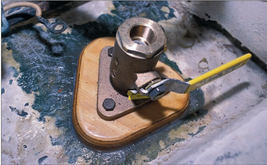
In this completed “aftermarket” seacock installation, the backing block is fully encapsulated in epoxy, and where the block adheres to the hull, all gelcoat has been removed. However, the bonding wire here is incorrect: it is solid, rather than stranded material, and was later replaced with stranded tinned cable.
