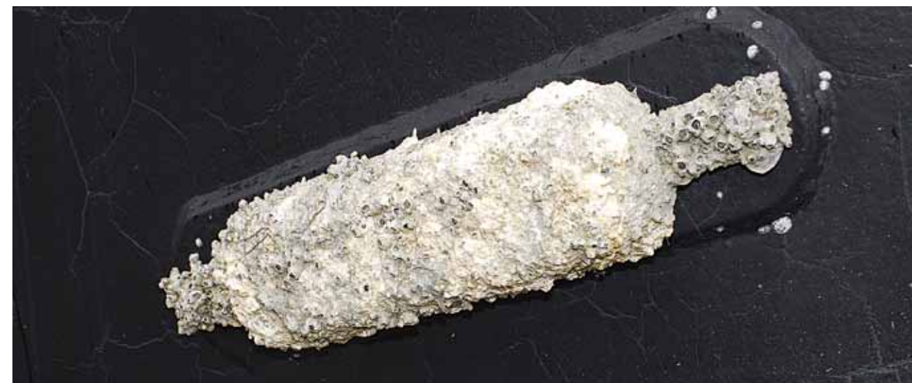
Top: Bonding system integrity should be checked periodically, especially if anodes are not being consumed or if they are being consumed unevenly. Above: When anodes are working properly, they should not become encrusted with marine growth.
