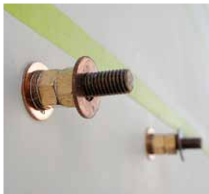
Left: Studs used to support anodes must be installed in such a way as to avoid relying on the anode to maintain tension.
