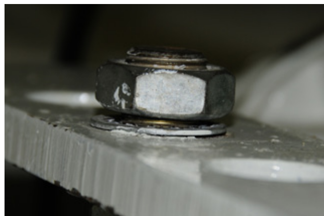
Loose motor mount locking nuts are especially common. Avoid using star (shown above), or split lock washers, instead rely on self-locking nuts or cam-style washers.
