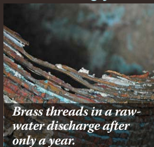
This brass pipe adapter crumbled after just a few seasons of use.
