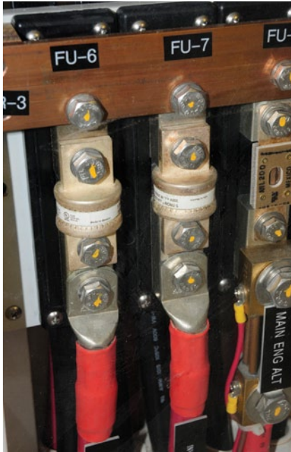
Class T fuses, like the cylindrical ones shown here, have a high amp interrupt capacity. These should be for power supplies from large battery banks and with most inverters.
