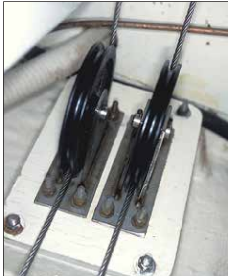
Precise cable-routing through multiple turning blocks is critical. If cables don't lie in the center of the sheave's groove, both will wear prematurely.
