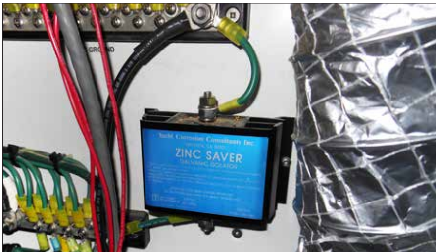
For vessels equipped with polarization transformers, an associated non-ABYC-compliant galvanic isolator does not meet fail-safe requirements and should be replaced with an up-to-date model.
