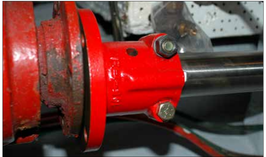
For good engine-to-shaft alignment, the significant angled gap between this shaft coupling and the transmission flange must be eliminated by compensating for shaft sag and then shifting the engine on its mounts laterally and adjusting the mounts vertically.
