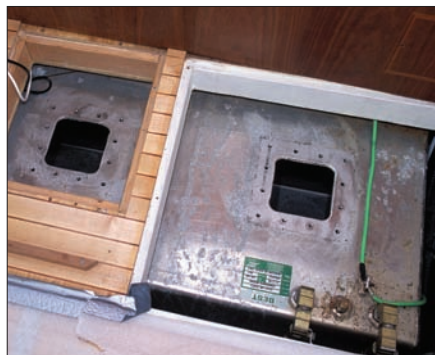
Fuel tank inspection ports are essential for monitoring diesel quality and condition. There must be one port in each baffled chamber of a connected fuel tank to allow thorough cleaning after contamination with bad fuel or bacteria.
