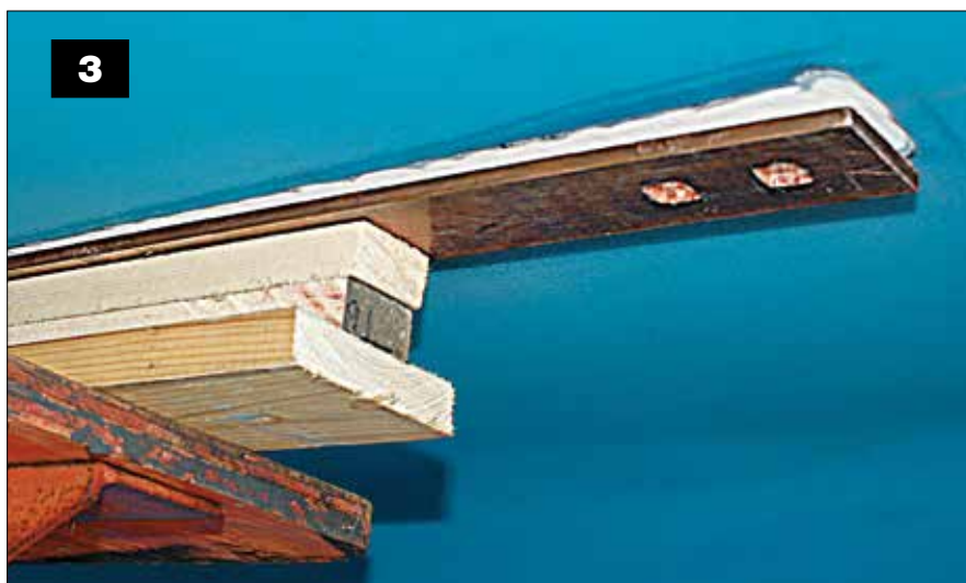
Dry-fitting a ground plate using shims and jackstands ensures that holes for through-bolt fasteners are exactly where they need to be. This long, narrow plate's square holes will engage carriage bolt fasteners.
