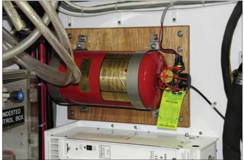
Fastened to the engineroom bulkhead on a secondary plywood panel, this bottle is secured horizontally.
