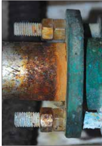
Corrosion of threads and shaft indicates a failure that may require adjusting or replacing components.
