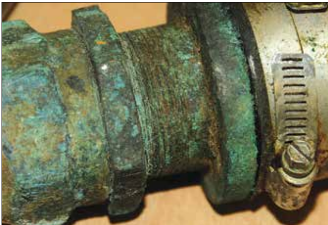
Inspect the stuffing box and associated hardware, including the hose clamps that seal the connection to the shaft log.
