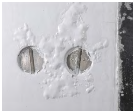
Minute flaws in coatings around fastener penetrations are common initiation points for corrosion of painted aluminum components.
