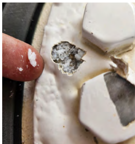
At breaches in the paint, water held against the underlying aluminum causes corrosion-forming aluminum hydroxide, a white byproduct.
