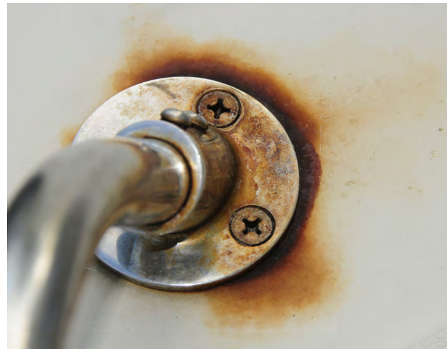
Deck hardware and fittings in 304 stainless steel are particularly vulnerable to "tea staining," where water can stagnate around fasteners and flanges. Cleaning and rebedding hardware is the best solution.
